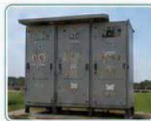
FEEDER PILLAR PANELS
