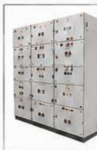
LT POWER CONTROL CENTER (PCC)
